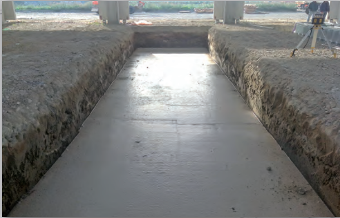
Fase 1: Preparazione platea a disegno. Stage 1: Excavation of the foundation to drawing 1 Phase: Vorbereitung der Grundplatte nach Plan
